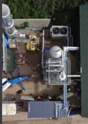
Photos showing the Hybrid WET plant in Warwickshire.
